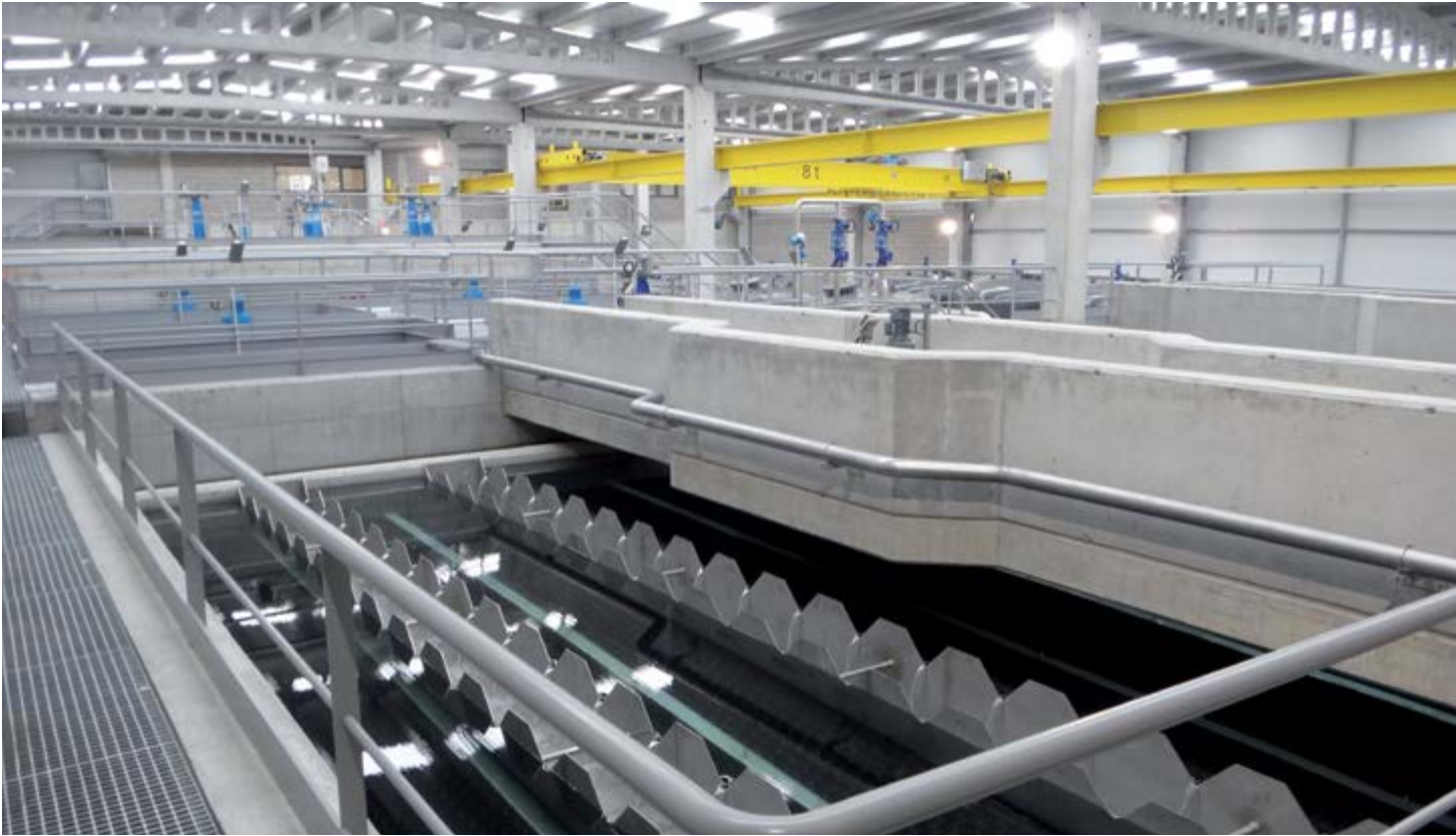
■ Drinkable Water Treatment Station (DWTS) of Monforte de Lemos, Lugo. Engineering and project: GSJ Solutions / Execution: SANJOSE Constructora
