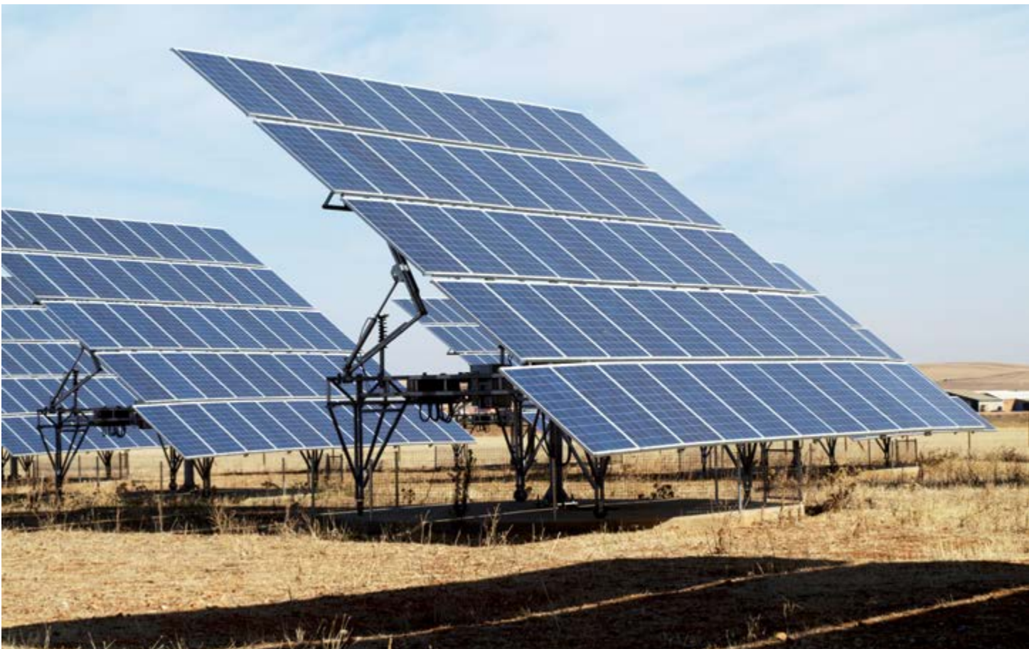
3.33 MW PV solar plant in Toro, Zamora
