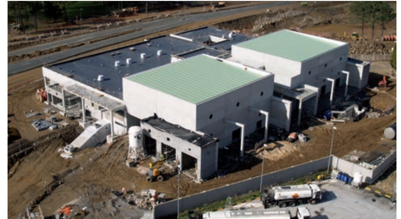
Electrical power plant at the Santiago de Compostela Airport
