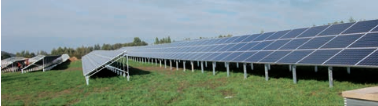
Photovoltaic power plant, Straz (Czech Republic)
