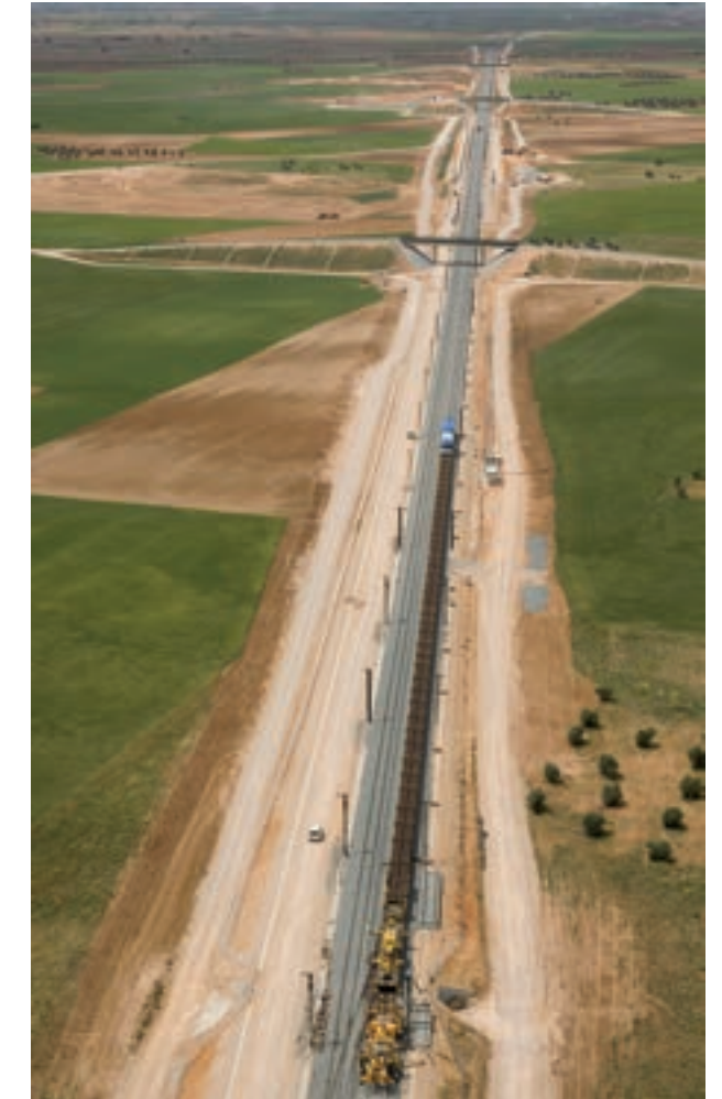
Stretch Ocaña - Villarubia de Santiago. Spanish National High speed Railway Network (AVE) Madrid - Valencia
