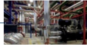
Polygeneration Plant in Cerdanyola del Valles, Barcelona
