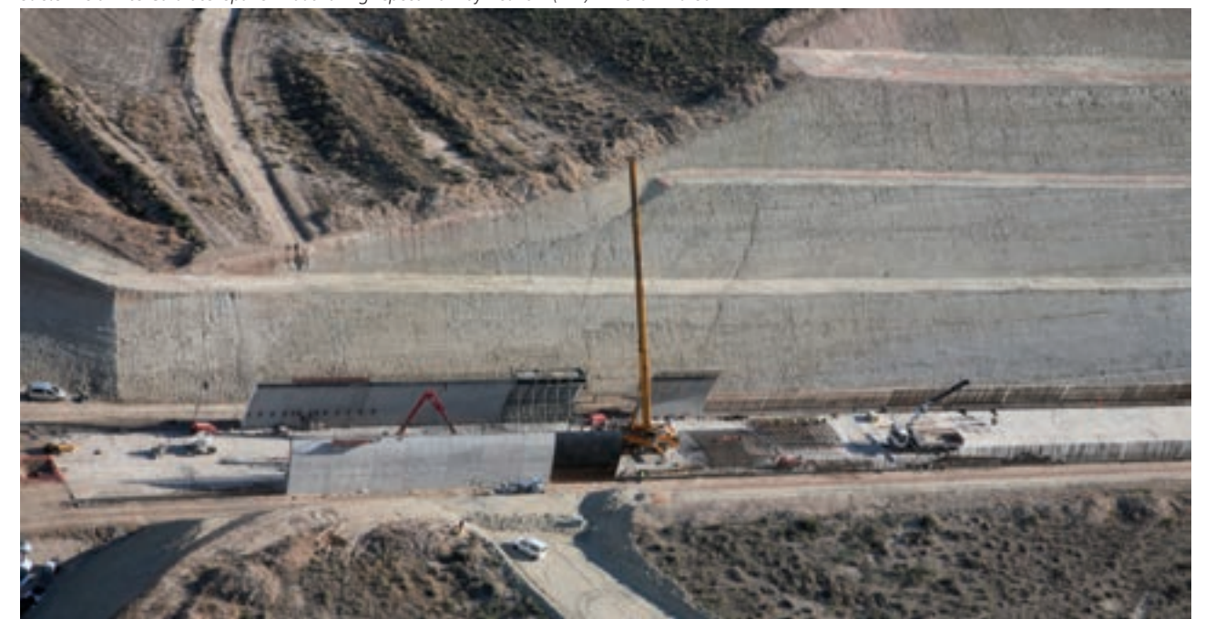
Stretch Vera - Los Gallardos. Spanish National High speed Railway Network (AVE) Almeria - Murcia
