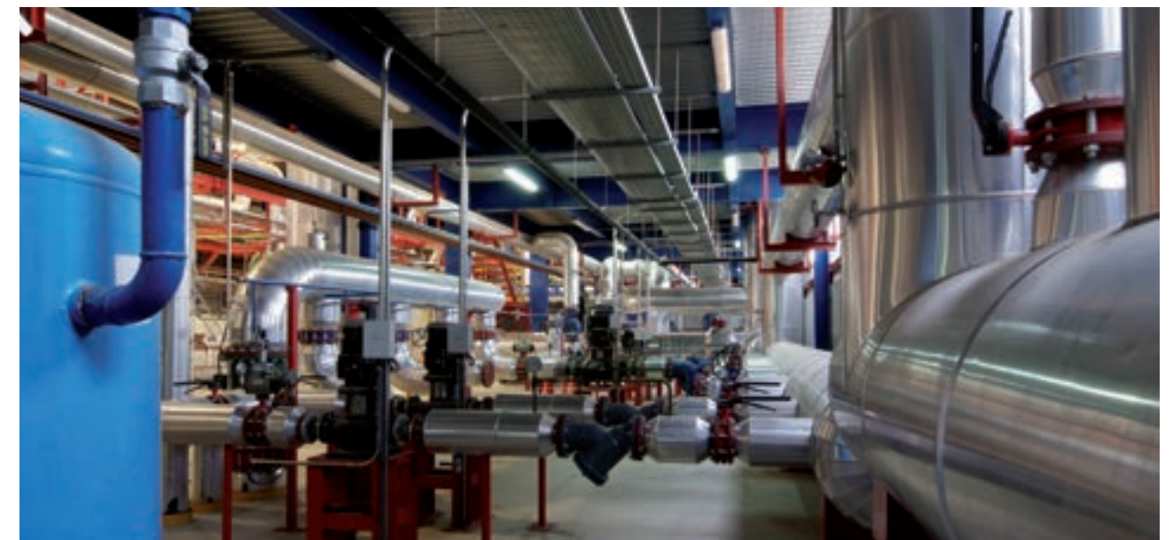
Energy supplier to the first Particle Accelerator in Spain and Southwest of Europe: Synchrotron Alba. Heating and Cooling Polygeneration Power Plant in Cerdanyola del Valles, Barcelona
