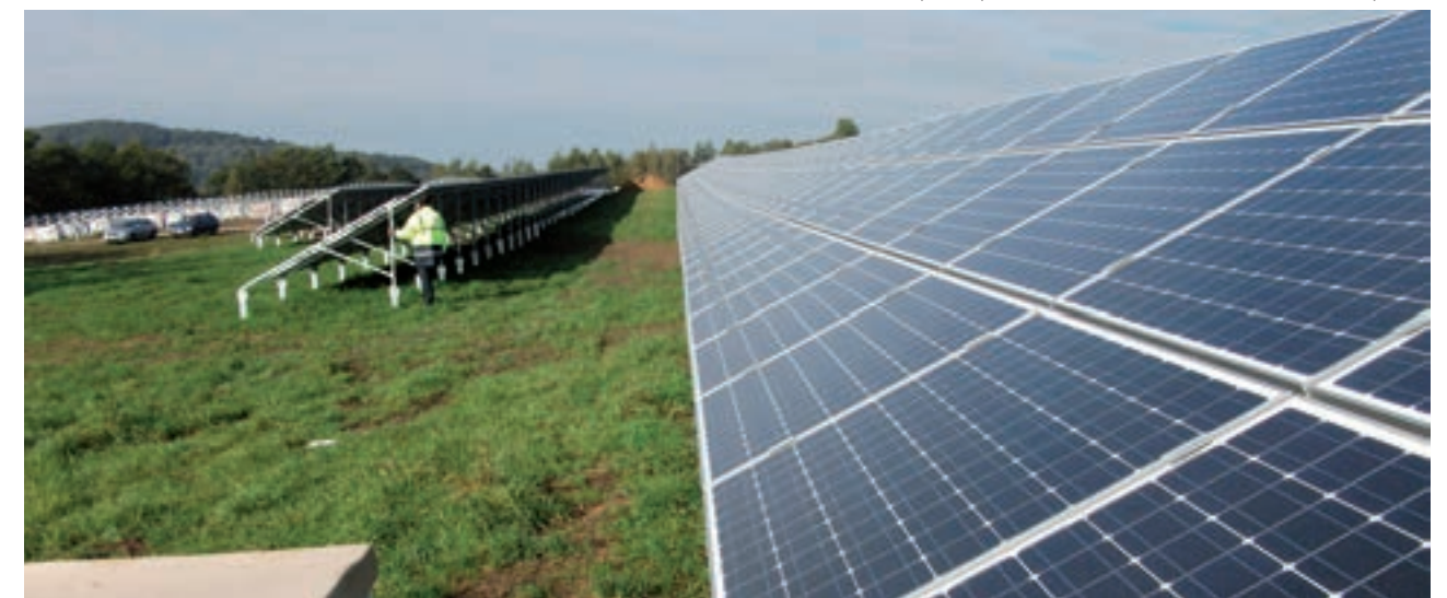
Photovoltaic power plant of 5 Mw in Straz Pod Ralskem (Czech Republic)
