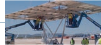
Maintenance of Photovoltaic Power Plants
