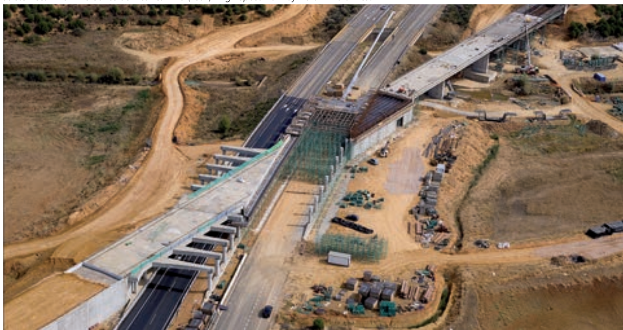
Stretch Cea River - Bercianos del Real Camino (Leon). High Speed Railway North - Northwest
