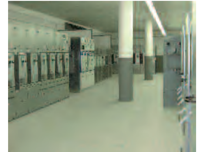
Electrical Substation, Anoia and el Bages.
