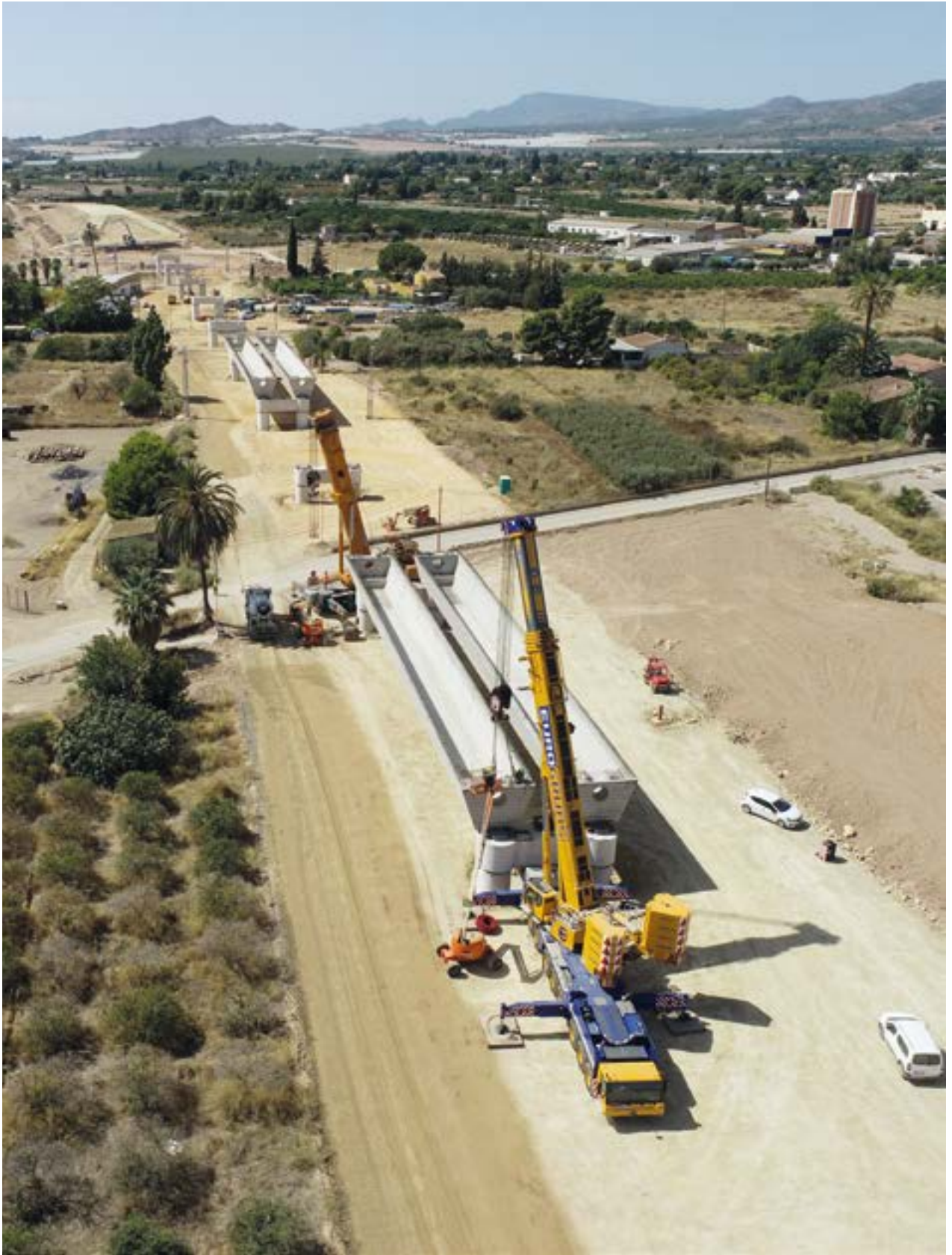
Stretch Sangonera - Totana of the Mediterranean High Speed Corridor Murcia - Almería (Spain)
