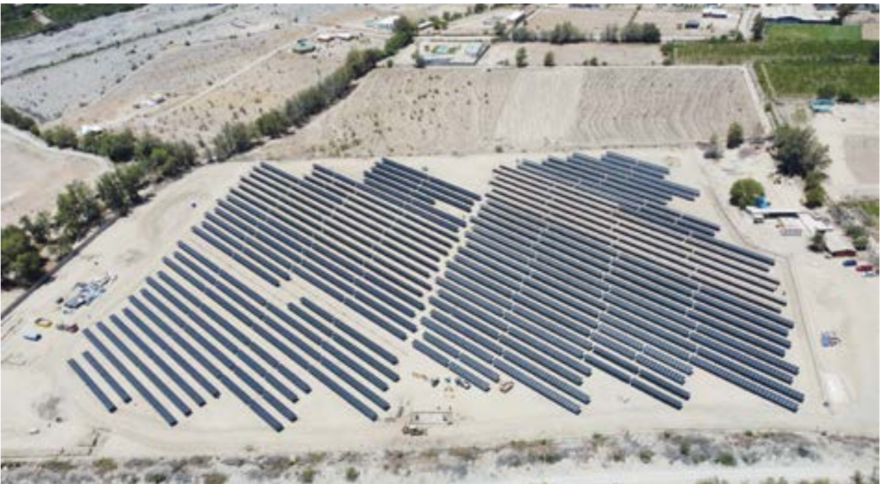
Olivier Photovoltaic Plant, Coquimbo Region (Chile). 3 MW
