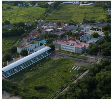
REFURBISHMENT OF THE GENERAL HOSPITAL ZONE # 5 IN ZAPATEC, STATE OF MORELOS (MEXICO)
