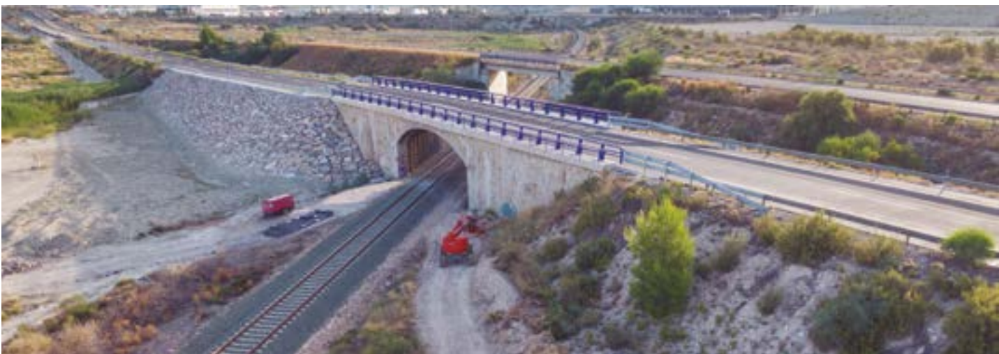
Repair of the bridge over the railway on the N-301 in Lorquí, Murcia (Spain)
