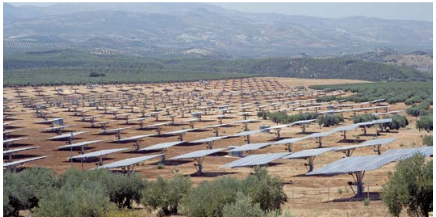
PV solar farm in Alcaudete, Jaen / 5,4 MW (Spain)
