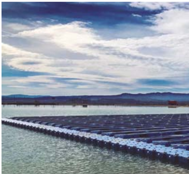
Floating solar pumping on raft and two underground pumps for self-consumption in the Irrigation Community of Llíria, Valencia (Spain)
