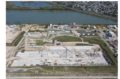
Expansion of the General Belgrano Water Treatment Plant, Buenos Aires
